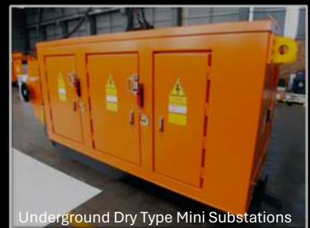
2MVA Dry Type Transformers
